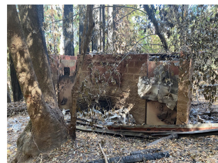
Burned restroom in the campground
